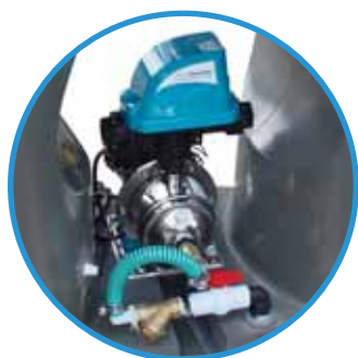
Pump installed behind inspection door
